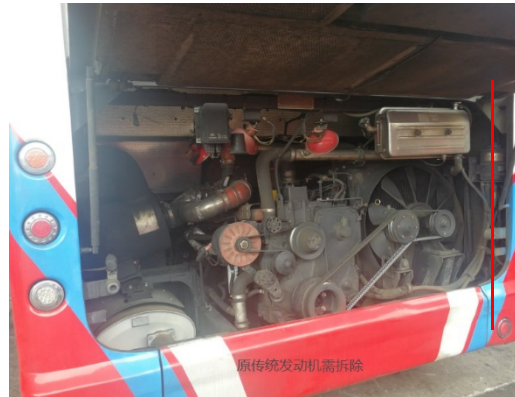
Conventional steering Liquid Storage tank
